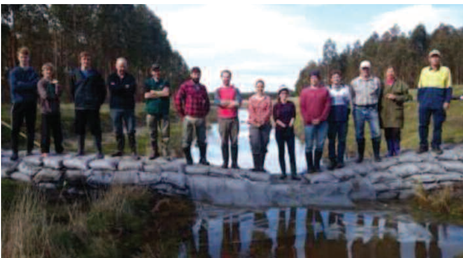
Staff and volunteers after completing construction of the sandbag weir they are standing on. Walker Swamp, Grampians, August 2014.
